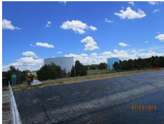
Figure 2-5 0.5 and 0.1 MG Tanks
